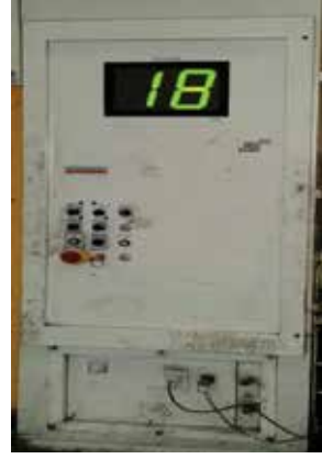
Yard. Operatör Paneli
